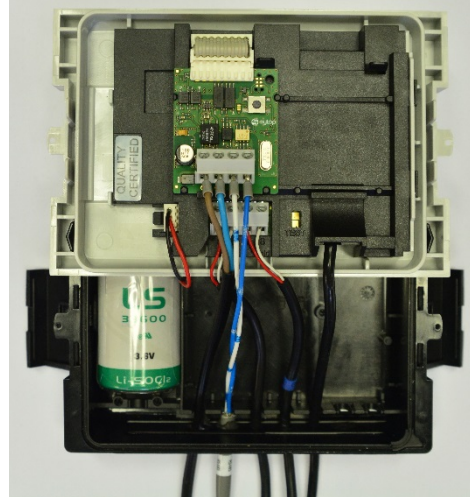
Picture 5.6 - Example of correctly wired module
